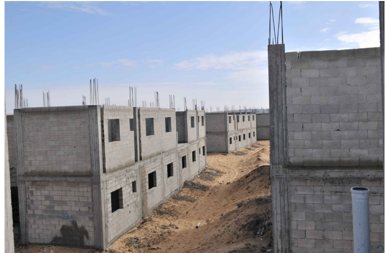
Partially finished units in the Khan Yunis housing project, frozen since June 2007 due to restrictions on the import of necessary materials. Photo by UNRWA
