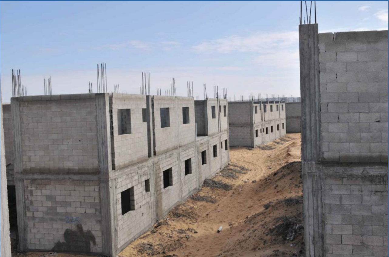
Partially finished units in UNRWA's Khan Yunis housing project. Photo by UNRWA.
